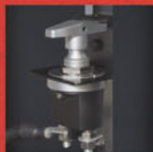
Lock. Battery Disconnect
